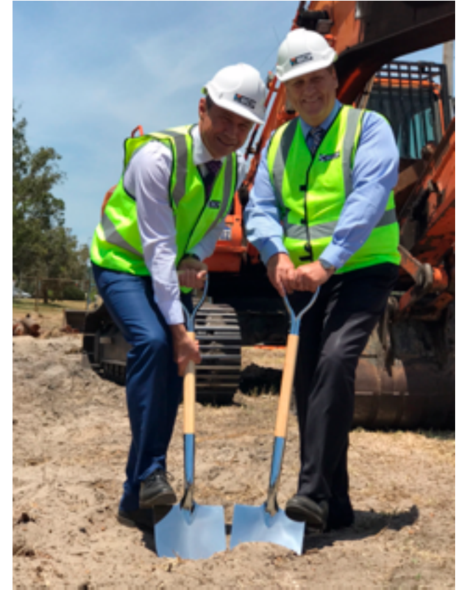
The Hon. Roger Cook MLA and Mr Donald Punch MLA, Member for Bunbury break ground at the site of the Bunbury Step Up/Step Down facility
